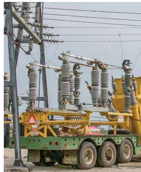
Upper Missouri's mobile substation transformer failed in July 2014. The mobile is being rebuilt and updated. Once repaired, Lower Yellowstone REA has indicated interest in owning, maintaining and managing the mobile substation and regulator.
