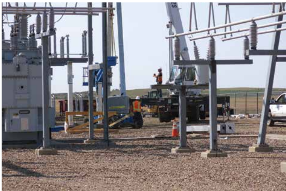
A new 115kV bay addition was completed at the Dickinson Substation to accommodate growth in the Dickinson area. Control upgrades were completed on the parallel regulation at Dickinson as well.
