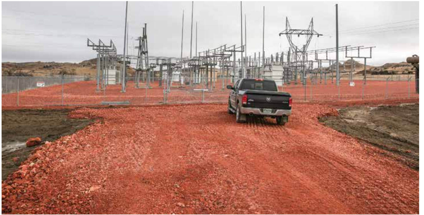
Major work was completed at Upper Missouri's Medora Substation in 2014. Structure/building stabilization, a new runoff control berm, and a new access road was developed in cooperation with the Teddy Roosevelt Medora Foundation and the U.S. Forest Service.
